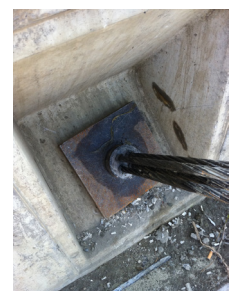
Recess in the concrete
