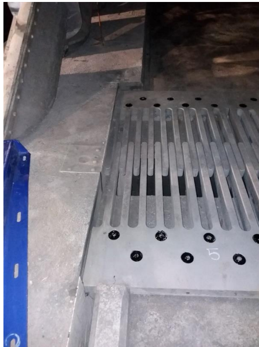
Figure 20 : Photo of a kerb cover plate
