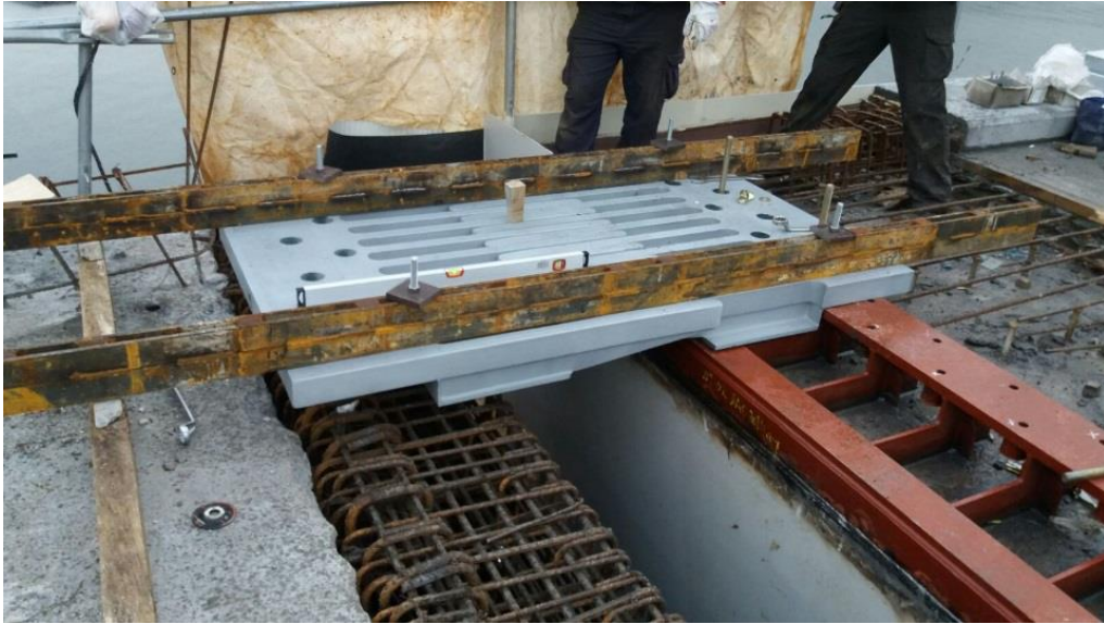
Figure 29 : Standard fixation on one side and special fixation on steel bridge on other side
